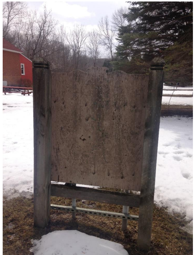
Back of Utility Box
