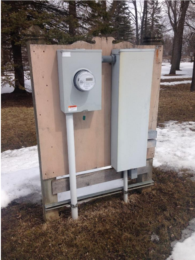
Front of Utility Box
